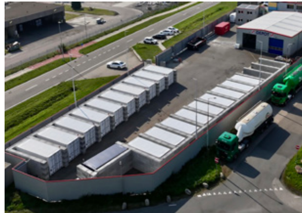
A&M Batteries Depot Humberweg
